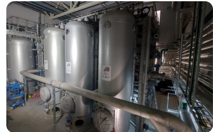
THP installed at Krogstad in Lillestrøm, Norway
