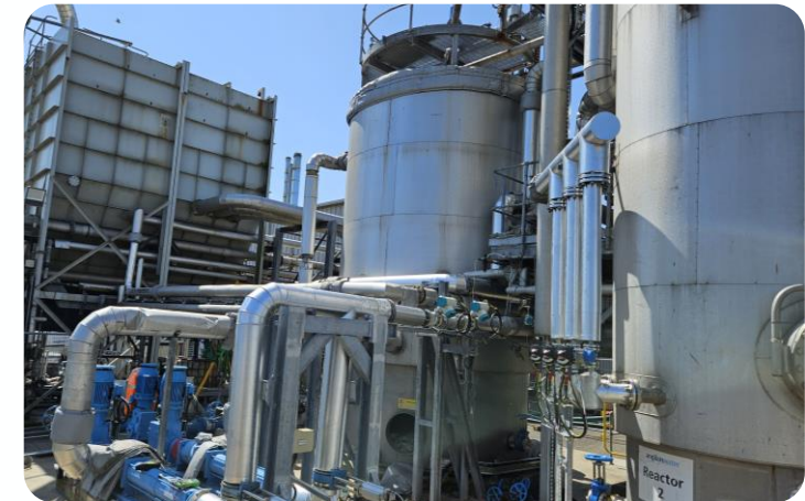
THP progressing through upgrade commissioning for Anglian Water at Whitlingham in Norwich, UK
