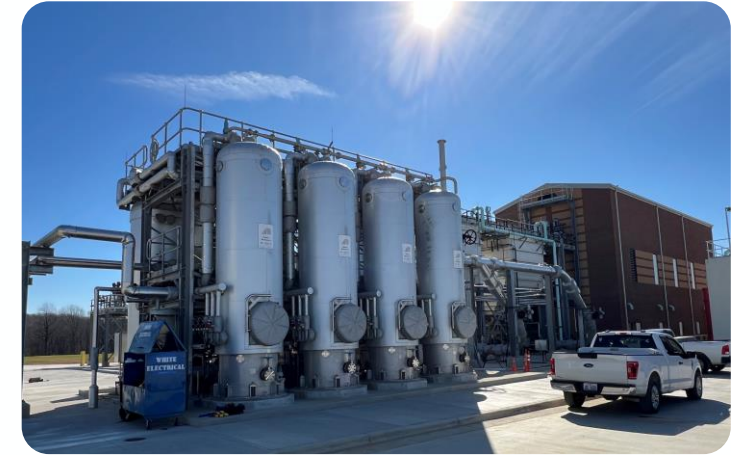
THP in operation at Neuse River RRF in Raleigh, NC
