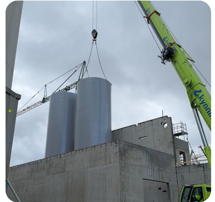
Sludge line taking shape in preparation for THP delivery at Øra WWTP in Fredrikstad, Norway
