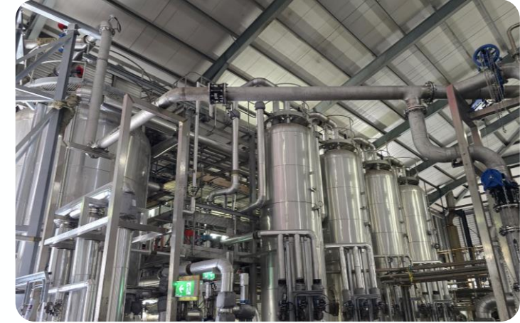
THP progressing through upgrade commissioning for Irish Water at Ringsend in Dublin, Ireland
