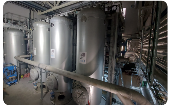
THP installed at Krogstad in Lillestrøm, Norway
