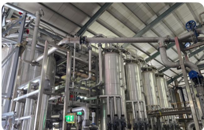
THP progressing through upgrade commissioning for Irish Water at Ringsend in Dublin, Ireland
