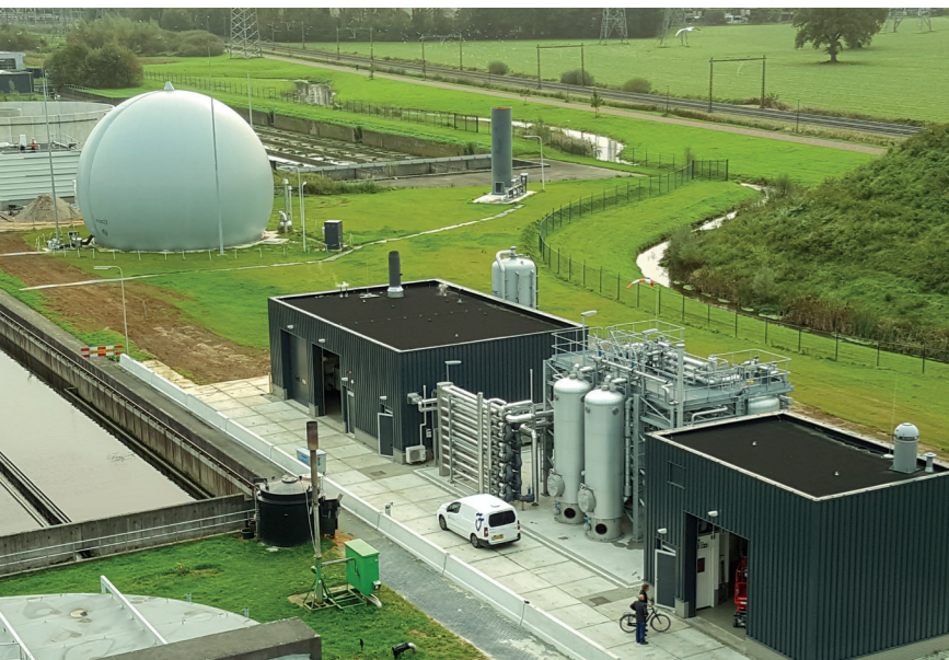
Cambi THP plant. Hengelo, The Netherlands.
