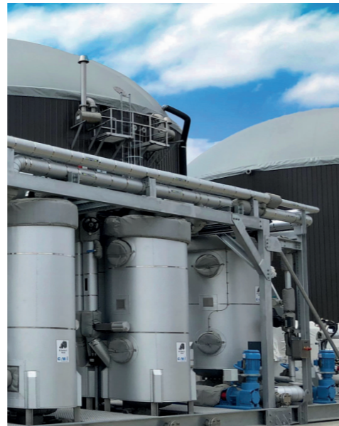
Cambi THP plant. Medina County, OH, USA.
