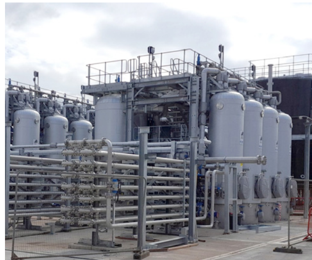
THP system commissioned at Finham WWTP, Coventry, England
