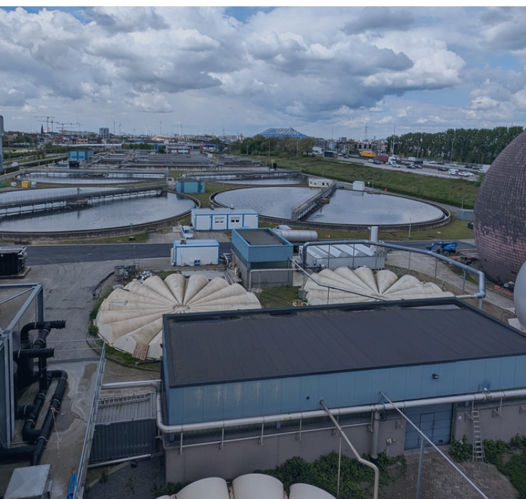
Deurne-Schijnpoort wastewater treatment plant in Antwerp, Belgium
