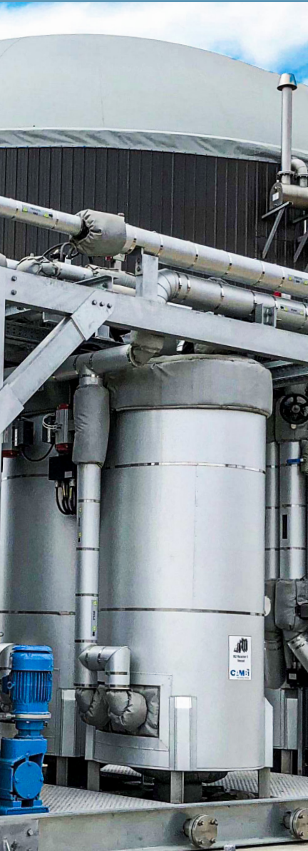
Cambi THP plant. Medina County, OH, USA
