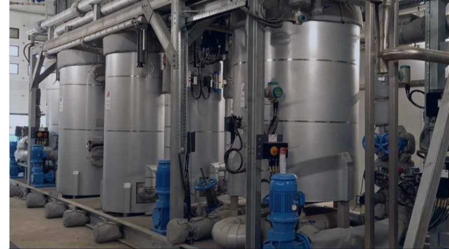
New THP in operation in Warsaw, Poland
