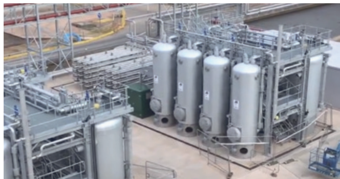
Minworth, the first Cambi THP plant for Severn Trent, Birmingham, UK
