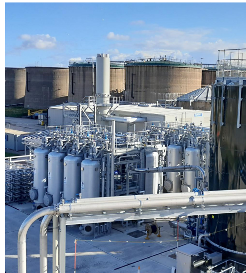
Newly commissioned THP system at Stoke Bardolph, UK
