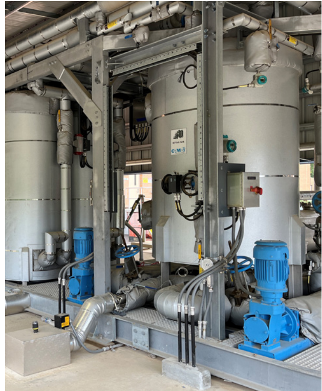
Cambi THP system in operation in Franklin, TN (USA)
