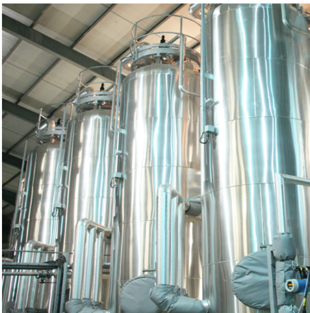
The third Cambi THP stream at Dublin's Ringsend WWTP (Ireland)
