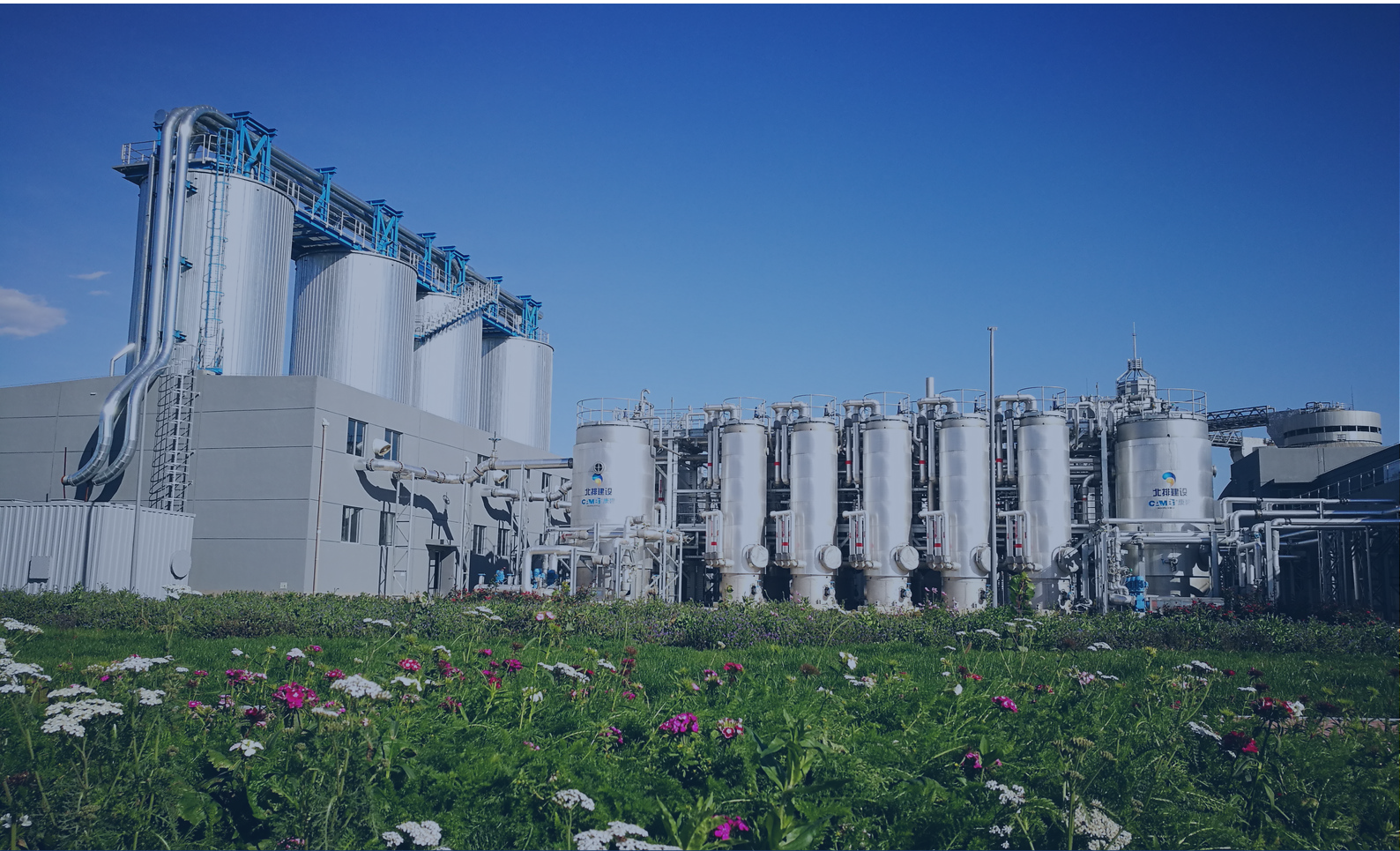
Large Cambi THP system in operation at Xiaohongmen wastewater treatment plant in Beijing, China
